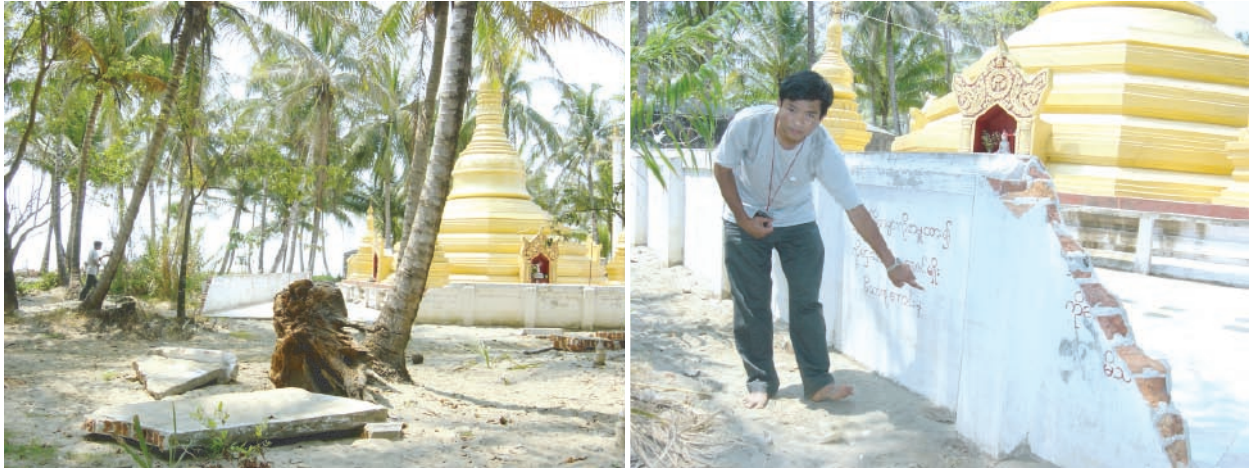
Photo 24. Field survey at Kaing Thaung Island Pagoda. Walls of Pagoda are destructed by Tsunami (left) and Watermark at the wall (right).
