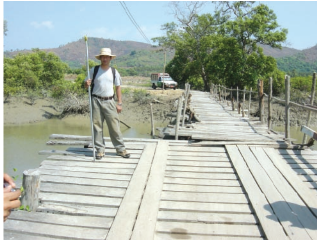
Photo 13. Destruction of bridge to Konnamaing Chaungwa Village by tsunami (narrow flat portion in the right far site of photo).
